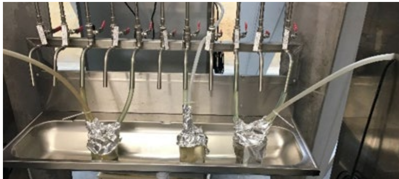
Figure 2.9 Sampling valve station for collecting grab samples.
