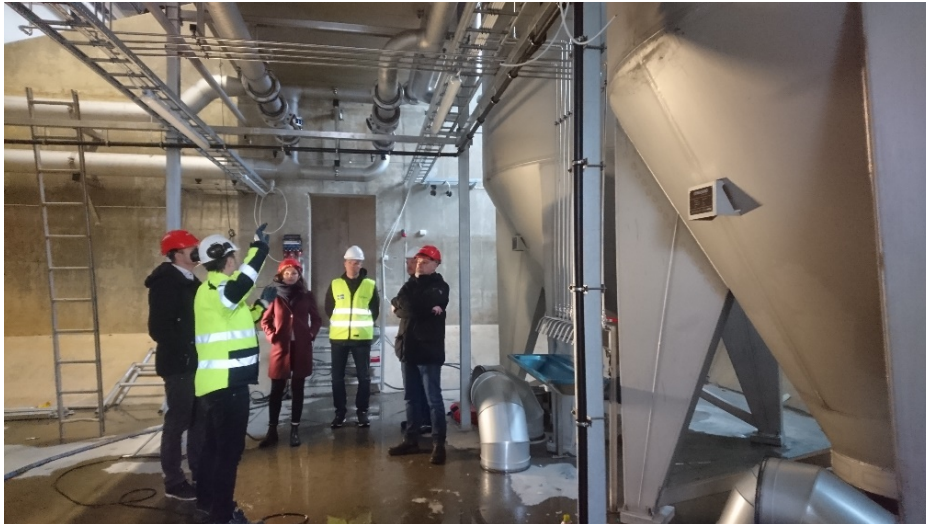
Figure 2.7 Two of the five Dynasand filters after installation
