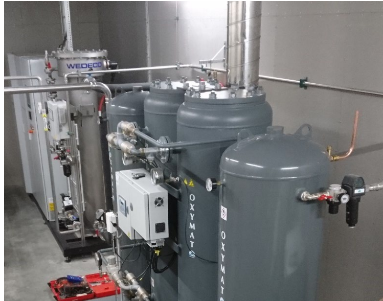
Figure 2.5 Full-scale installation of the ozonation system.
