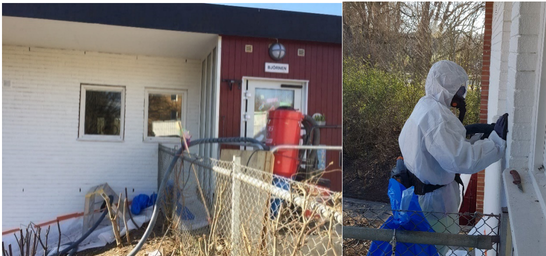
Figure 7. An example of sanitation work at a kinder garden in Lund. Window frames from the 50's containing PCB materials and cannot be reused. Ref: IVL
